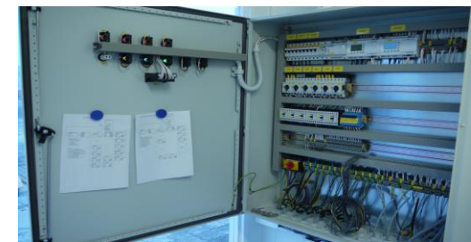
control cabinet on technical container
