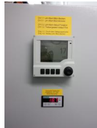
adjustment switch cabinet dosing pump
